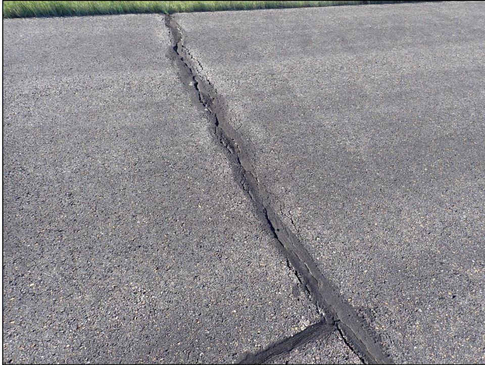
RW07-03-05: L&T Cracking
