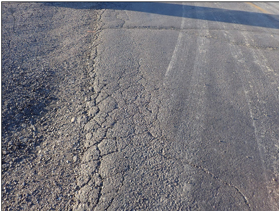
TW-03-02: Alligator Cracking
