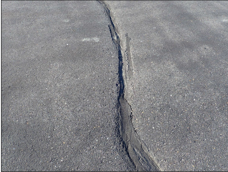
AP-05-07: L&T Cracking
